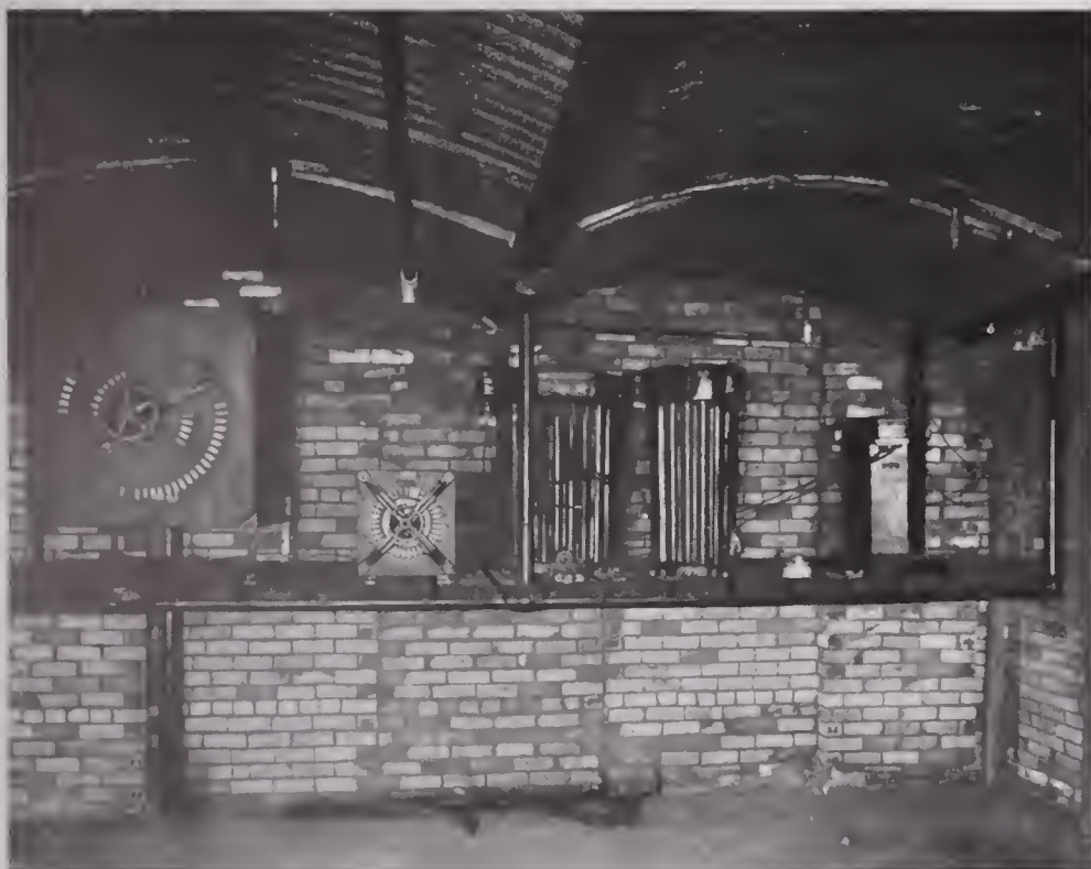
RHEOSTAT AND TRANSFORMER RACK
